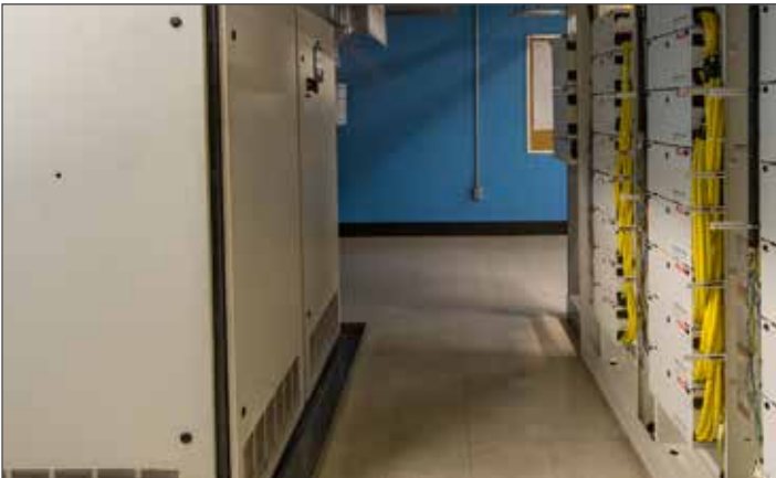
fiber distribution panels/meet me area
