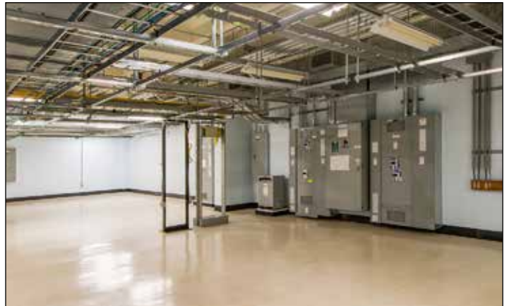
available floor space for racks, cabinets and cages
