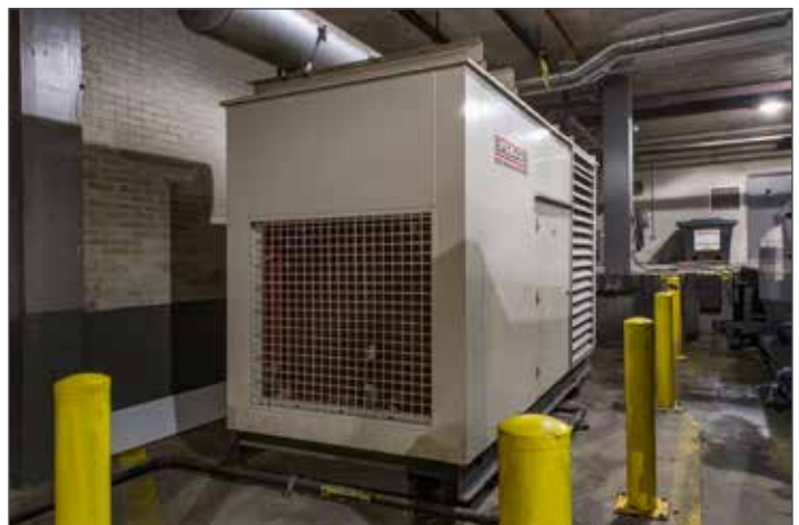
natural gas-powered backup generator
