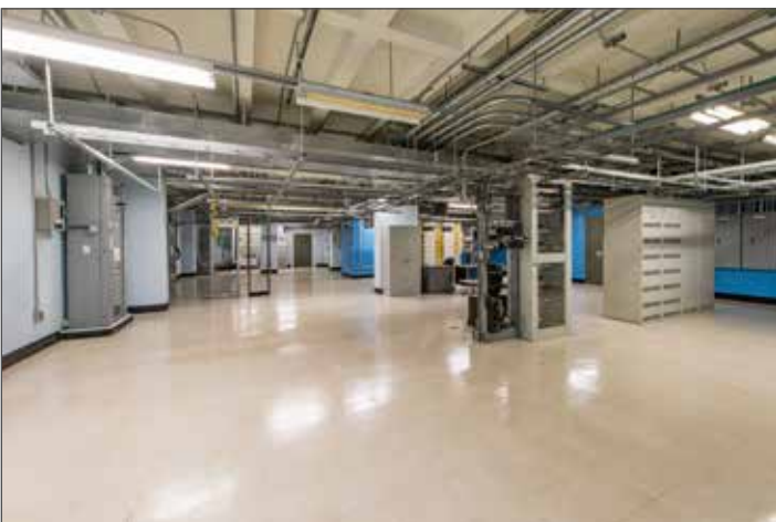
available floor space for racks, cabinets and cages
